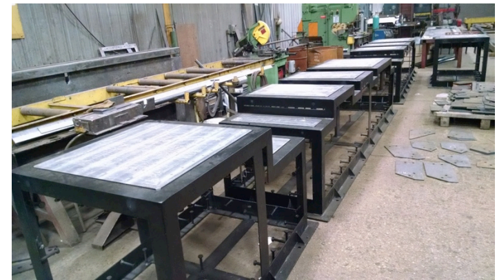
Steel frames for the Plinth R&D at Corsetii Steel. Concrete pouring will take place next week at Dukane Precast.
